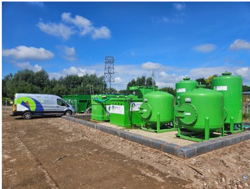
Oracle Environmental Experts water treatment system installed on a housing development in the Midlands
